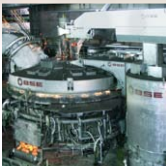
Electric Arc Furnaces
