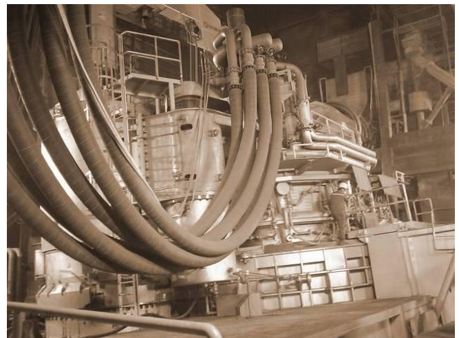
One of the revamped twin-shell furnaces at Posco Gwangyang Works, Republic of Korea
